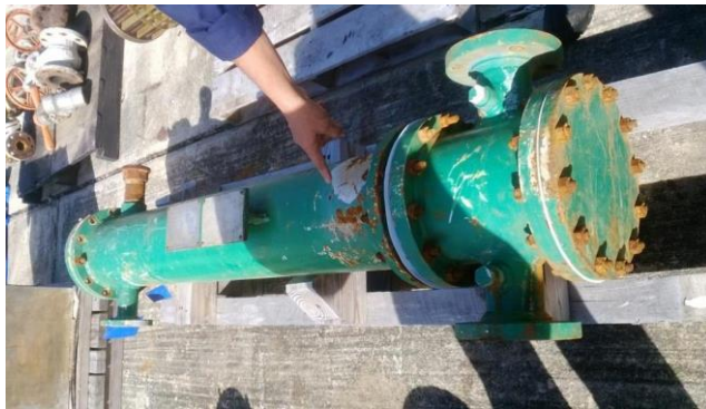
Gambar 52. Heat Exchanger Shell & Tube Terpasang di Kamar Mesin.
