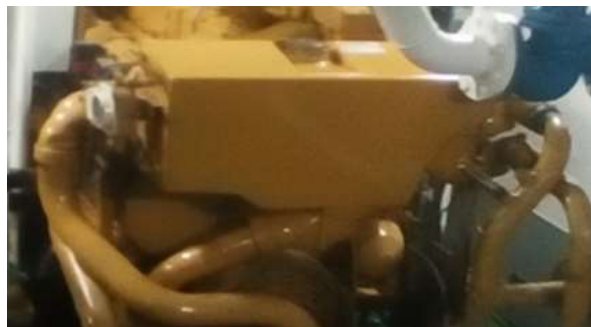
Gambar 1. Fresh Water Cooler
