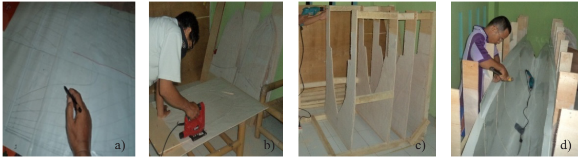
Gambar 4. Pembuatan cetakan luar core lambung perahu. Figure 4. Making the outside molds of the boat hull core.
