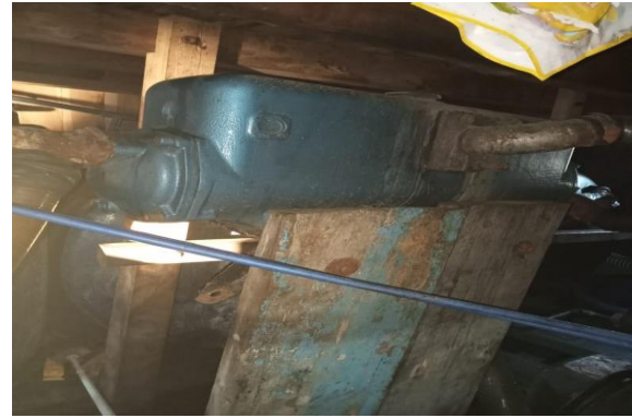
Gambar 4. Cooler Figure 4. Cooler Sumber: Pribadi
