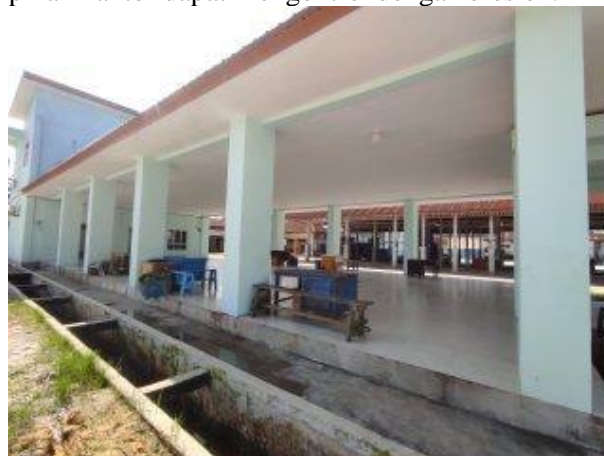
Gambar 3. TPI Tampak Samping Figure 3. TPI side view Sumber: Hasil penelitian
