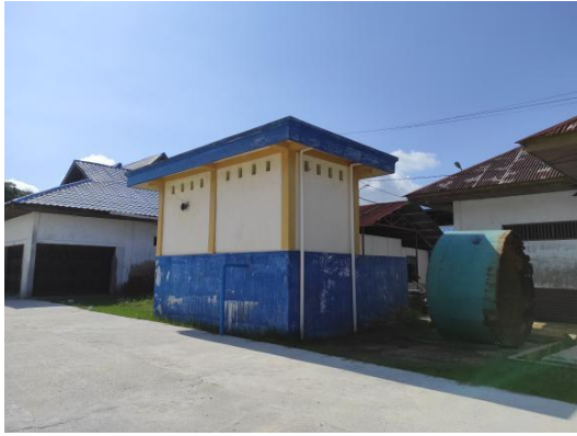
Gambar 13. Sumur bor Figure 13. Boreholes Sumber: Hasil penelitian
