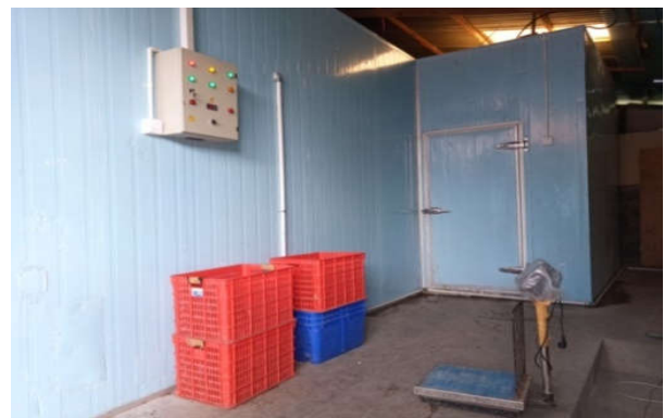
Gambar 5. Gudang Pendingin (Cold Storage).
