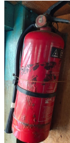
Gambar 5 Alat Pemadam Api Ringan (APAR) Figure 5 Light Fire Extinguisher
