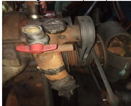
Gambar 6. Pompa Air Tawar
