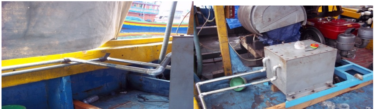
Gambar 10. Pemasangan sistem perpipaan minyak hydraulic di atas kapal uji Figure 10. Installation of the hydraulic oil piping system on the test ship
