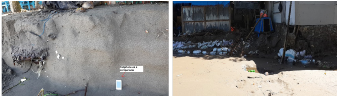
Figure 4. Steep sand dune and derelict semi-permanent structures as evidence of beach erosion in Pangandaran.
